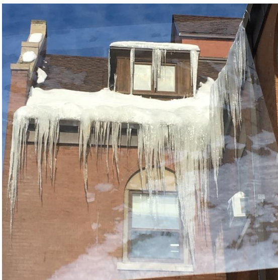
Babcock Roof Lack of Insulation & Venting
