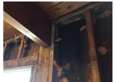
Northwestern Apartments - Mold and Dry Rot
