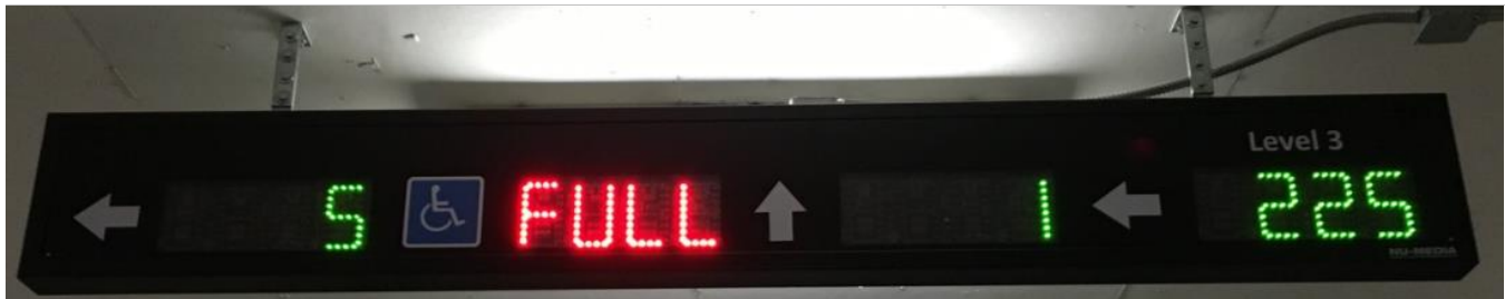
Figure 15: End of Aisle Space Availability Sign.
