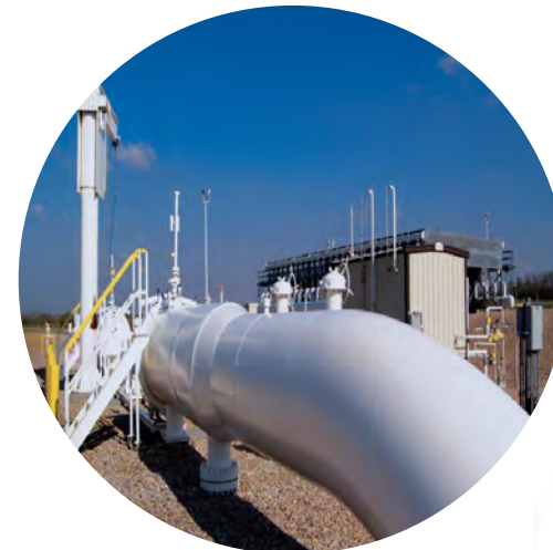
Natural Gas Pipeline Blending
