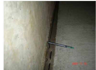
FAILED JOINT SEALANT
