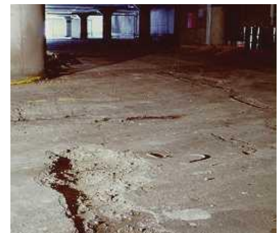
EXTENSIVE FLOOR SLAB SPALLING
