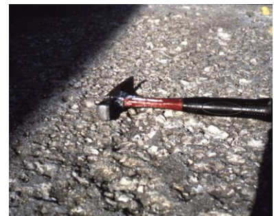
HEAVY SURFACE SCALING
