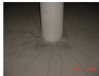
CRACKS RADIATING FROM COLUMN
