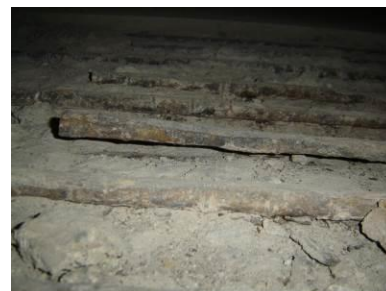
CORROSION OF REINFORCING STEEL IN FLOOR SLAB
