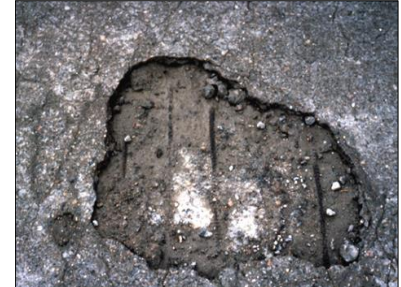
CORROSION INDUCED SPALLING IN FLOOR SLAB
