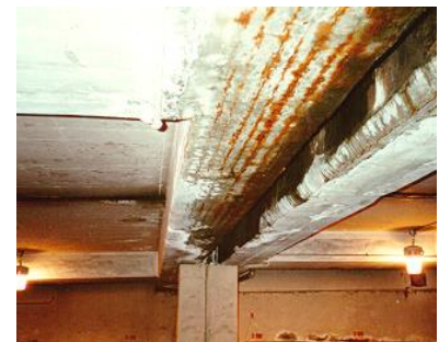
CORROSION OF REINFORCING STEEL IN/THROUGH CONCRETE BEAM
