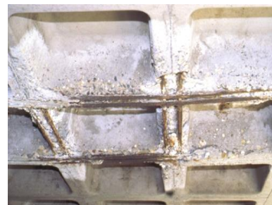
CORROSION INDUCED SPALLING AT UNDERSIDE OF WAFFLE SLAB
