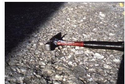
HEAVY FLOOR SCALING
