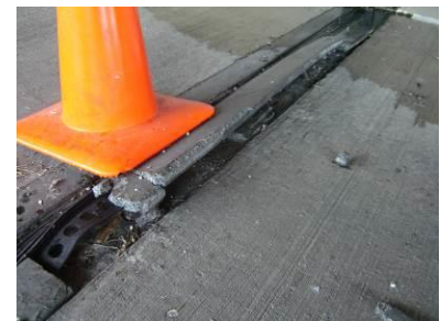
FAILED EXPANSION JOINT
