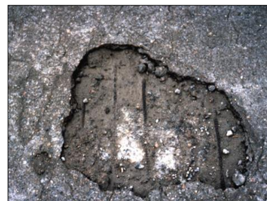
CORROSION INDUCED SPALLING IN FLOOR SLAB
