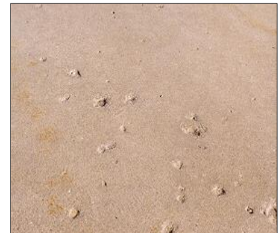
FLOOR SLAB POPOUTS
